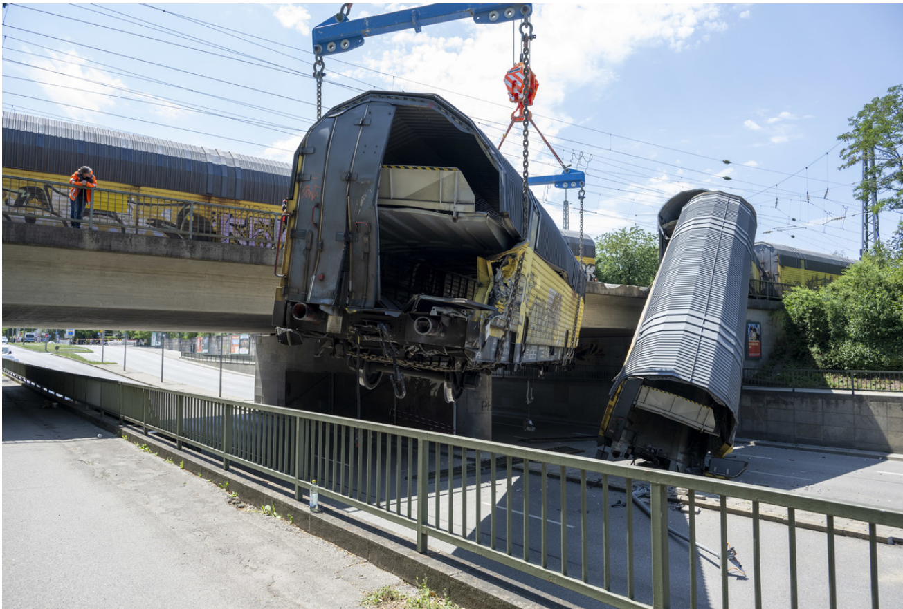
Rescue operations seen underway for two railcars of a freight train after falling from a bridge, June 19, 2026, Munich, Bavaria, Germany. © Stefan Puchner/picture alliance via Getty Images
