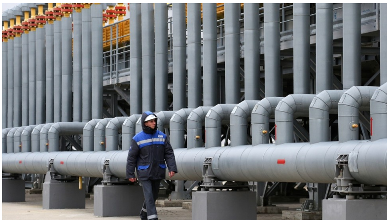
FILE PHOTO. Russkaya compressor station, part of the gas pipeline system that supplies gas to the Turkish Stream. Krasnodar Region, Russia. © Getty
